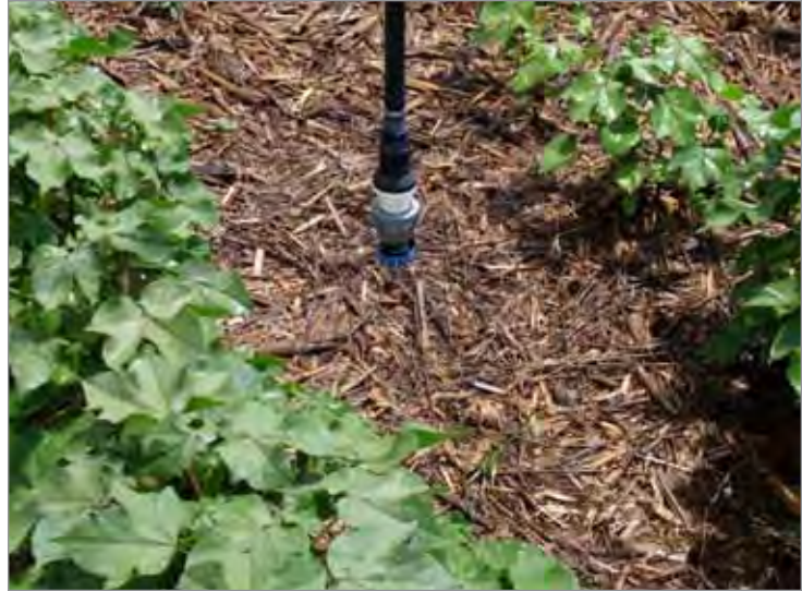
Figure 0.1 – Drop line from a center pivot providing water to a minimal tillage cotton field.
