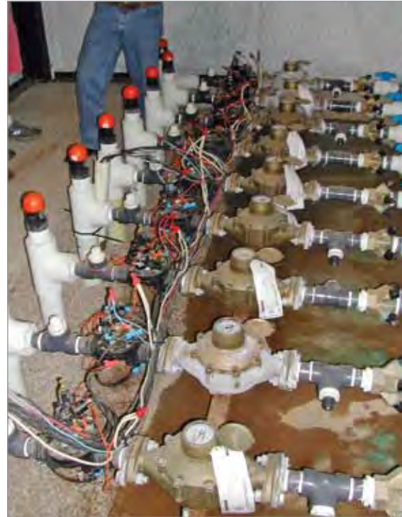
Valves controlling water delivery to different drip irrigation sections
